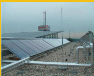
Solar thermal collector (surface 70 m 2 ) at OÖ Ferngas building in Haid (Source: OÖ Ferngas AG)
